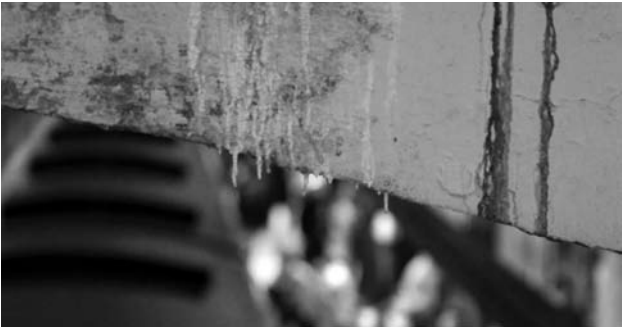
Top) The Guy-Concordia metro is coming to pieces around the Concordia students who use it. Bottom) The metros are filled with mold, decay and the homeless. Little has been done to improve the condition of our public transportation system.
